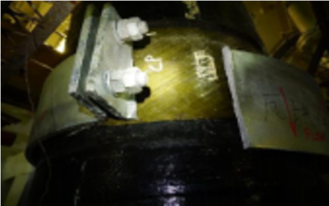
Detached seawater outlet pipe
