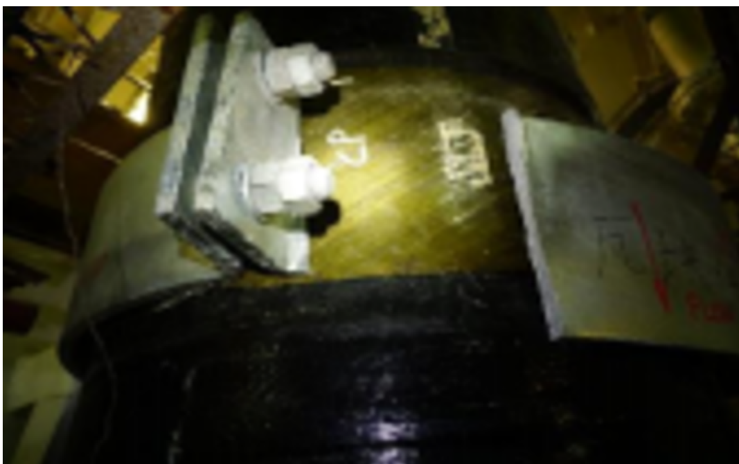
Detached seawater outlet pipe
