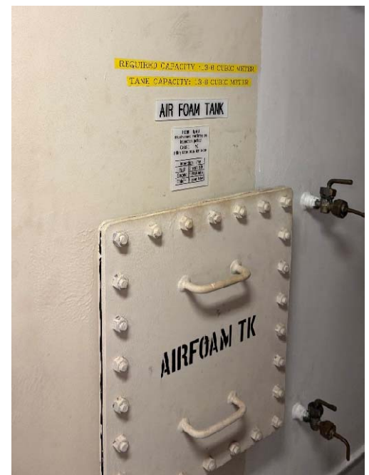
Foam storage tank – determines system endurance
