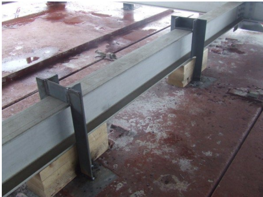
Steel brackets welded to the deck securing a purposely made frame supporting project cargo Note anti-slid timber beams sections placed underneath the frame
