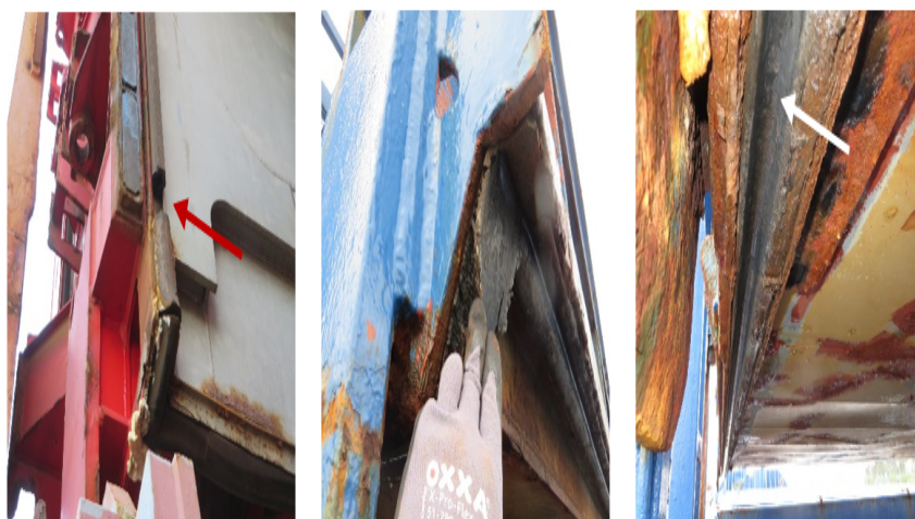
Gaps between insert repairs
