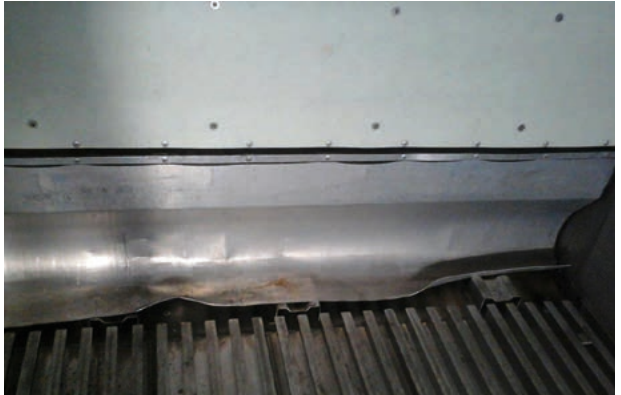
Picture 13 Damage to machinery airflow baffle.
