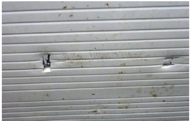
Picture 8 Cargo or forklift truck mast damage to the aluminium ceiling panels.
