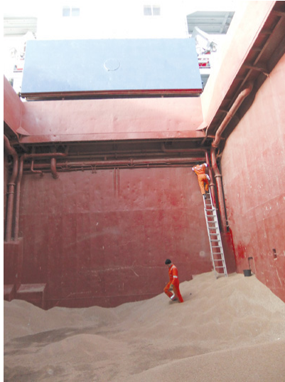
Aft bulkhead of cargo hold No. 3. The ventilator opening is in the corner, above the ladder. Access is difficult, as it is behind pipes under deck.
