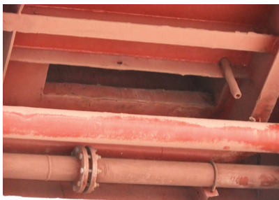
Ventilator opening in deck at the aft bulkhead of cargo hold No. 3. The steel bulkhead is the common boundary between the accommodation and the cargo hold ventilator.
