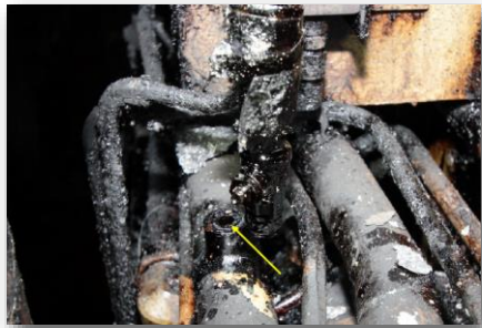
Why did the connection fail?
